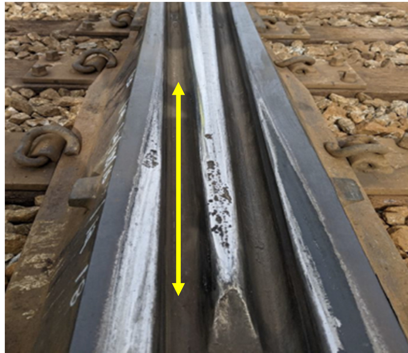
With 24" x 1/8" wing slopes: Nortrak WBM frog with heavy point, flat top profile (135 MGT); wheel tread contact on wings begins much closer to point.
